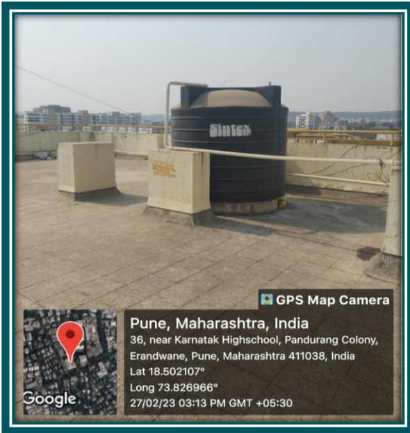
Overhead water tank
