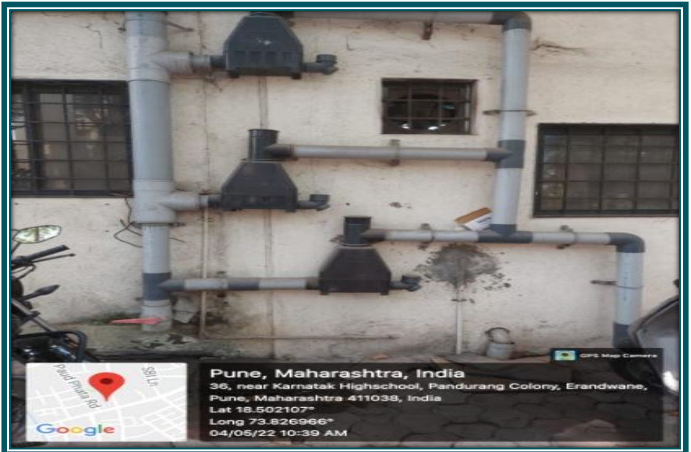
Rainwater Harvesting System
