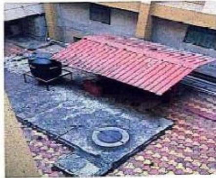
(Rooftop Rain Water Harvesting System)
